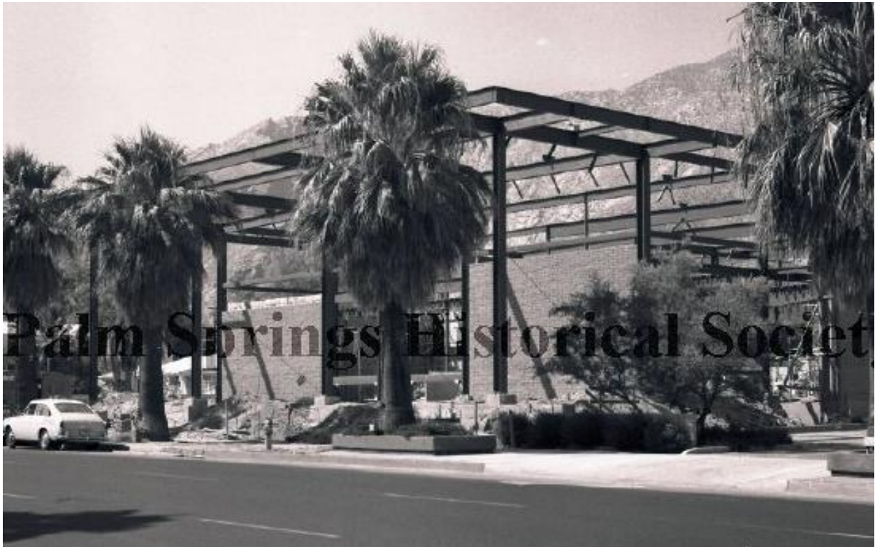
This photograph taken during construction shows the steel-framed building's structure. Courtesy Palm Springs Historical Society.
