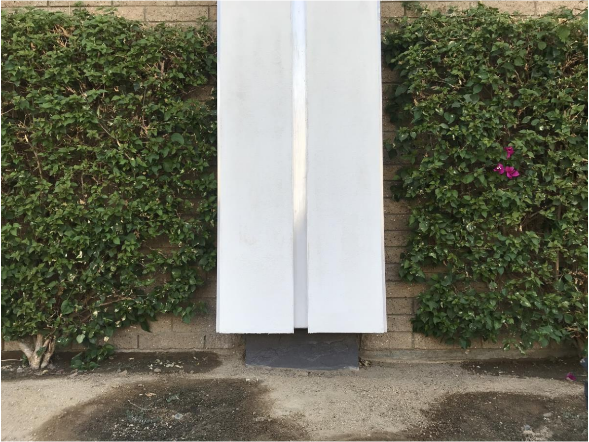
One of the squared embedded columns, created with off-white-painted plaster, embedded with a brushed aluminum “U”-channel. Note the dark-painted smaller blocks, which are at the top and bottom of the columns, giving the illusion of weightlessness. Photograph by the author June 2022.
