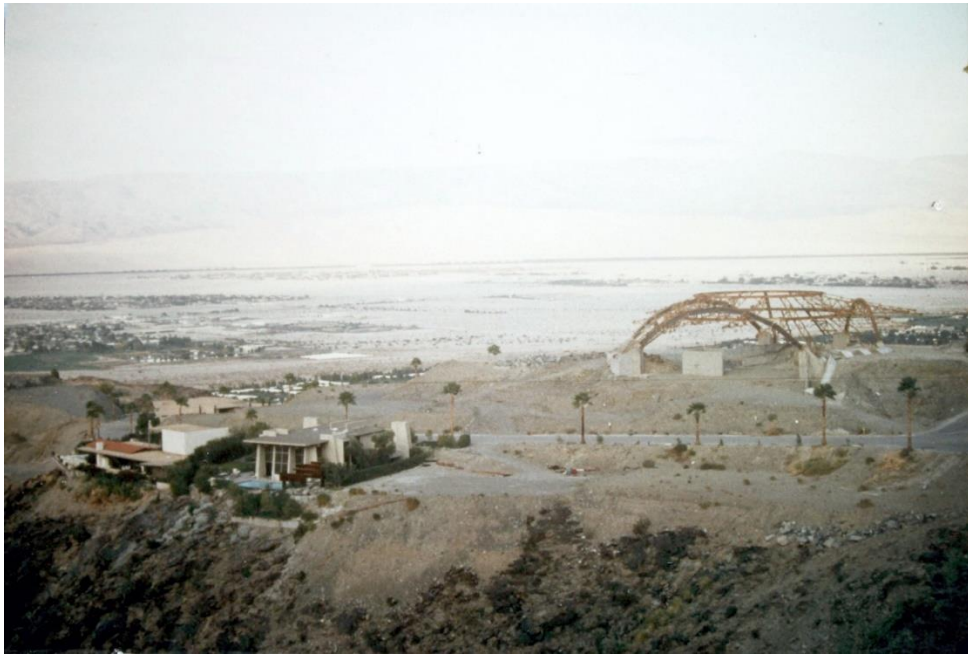
December 1975 – The Bob Hope House under construction, with Garber Residence in foreground at left.
