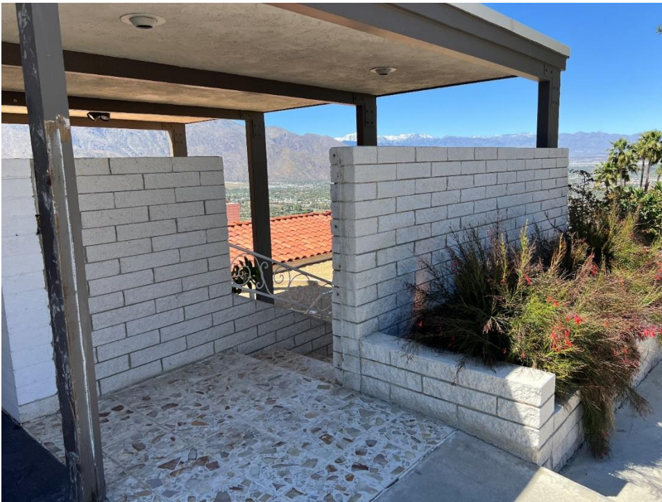
The stairs leading from carport area below to entry. Post-and-beam over off-white split-face concrete block. Floor is terrazzo tile.
