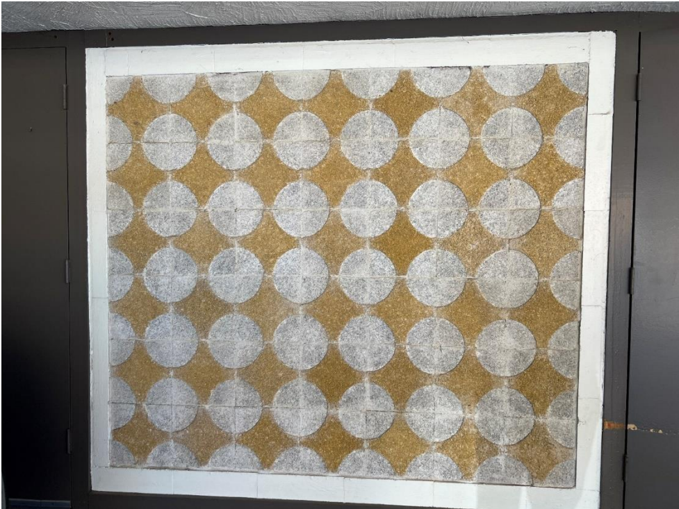
The rear wall of the carport features a geometric decorative panel created using tiles made from marble chips.
