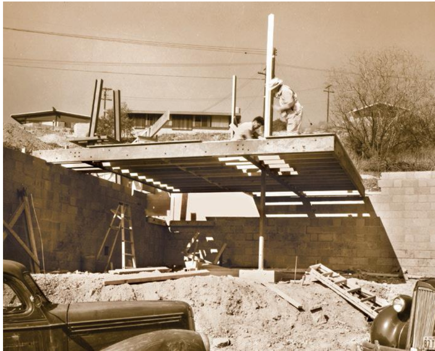
Crestwood Hills in Los Angeles while under construction in the late 1940s.
