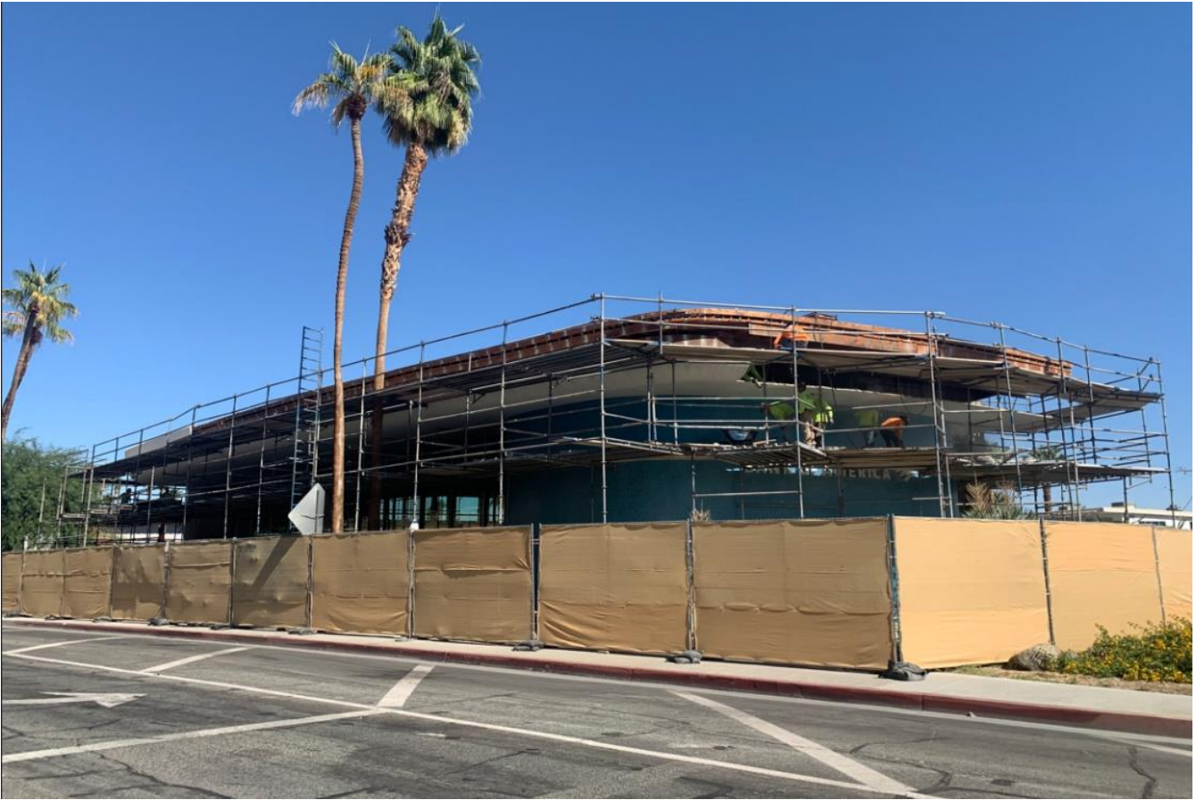
Exterior renovation at 588 S. Palm Canyon Drive circa 2023. Photo Credit: Gary Johns, President, Palm Springs Preservation Foundation Board of Directors
