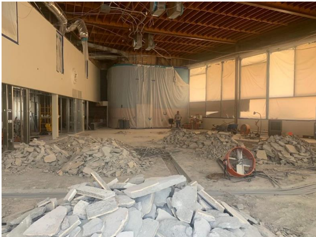
The interior of the Bank of America building was completely demolished during the building's restoration. (Photo courtesy Gary Johns)
