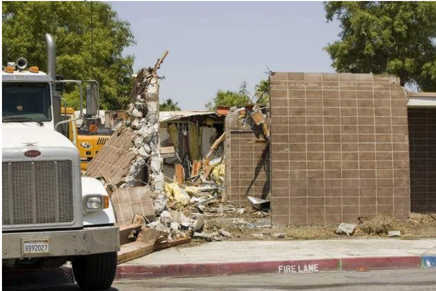
A building attached to the Palm Springs High School, which was designed by Donald Wexler, is being demolished on Monday, August 20, 2012. / Omar Ornelas, The Desert Sun
